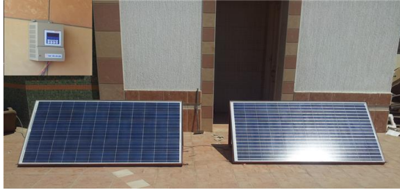
Fig. (14) Total PV experimental system
