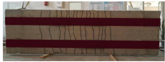
Fig. 22: Cracks pattern for S2ST2 at p=190 kN
