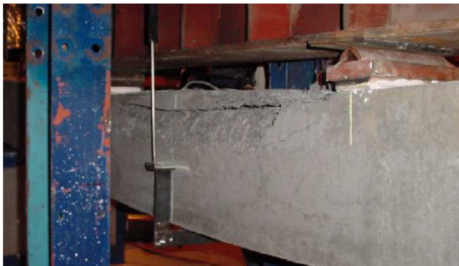
Fig. 4 Concrete cover spalling off for beam 12HP25
