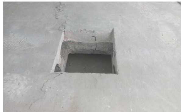
Fig. 12: Cracks pattern at top surface for PPHCS2
