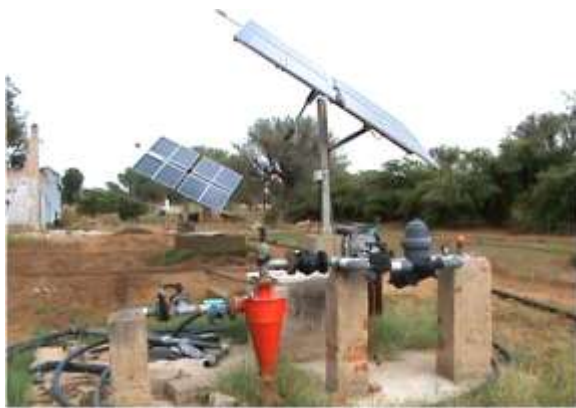
Fig.11. The existing PV pumping system at the site
